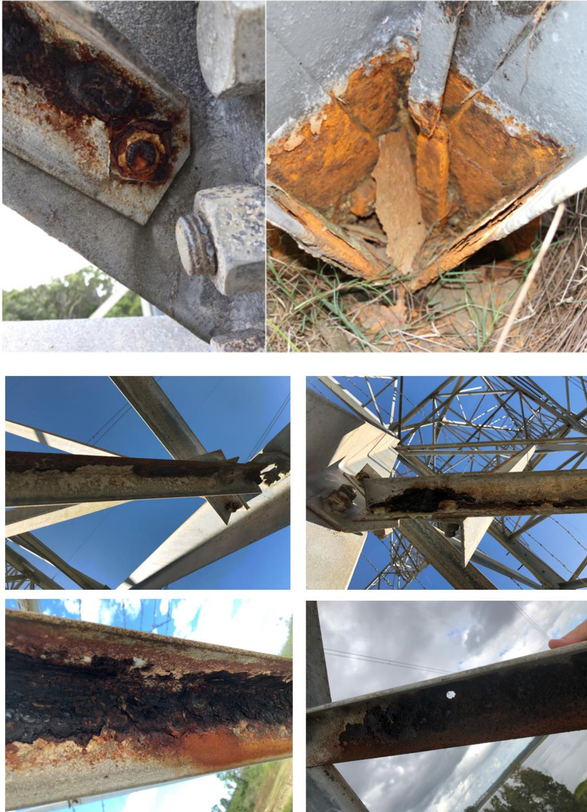
Figure 2-4 Examples of corroded components of Line 25 and Line 26: transmission tower steelwork and legs
