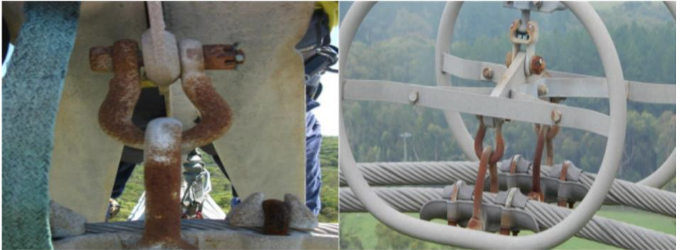
Figure 2-3 Examples of corroded components of Line 25 and Line 26: earthwire and conductor fittings
