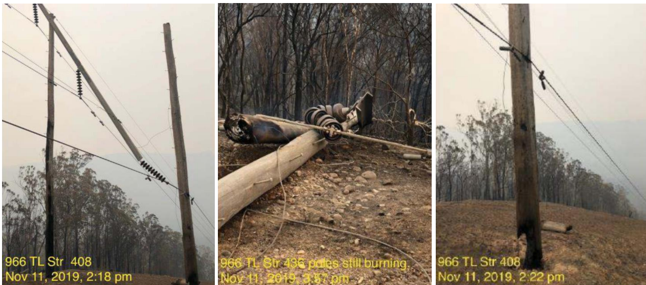
Figure 2-2 Damage caused to Line 966 in the November 2019 bushfires
