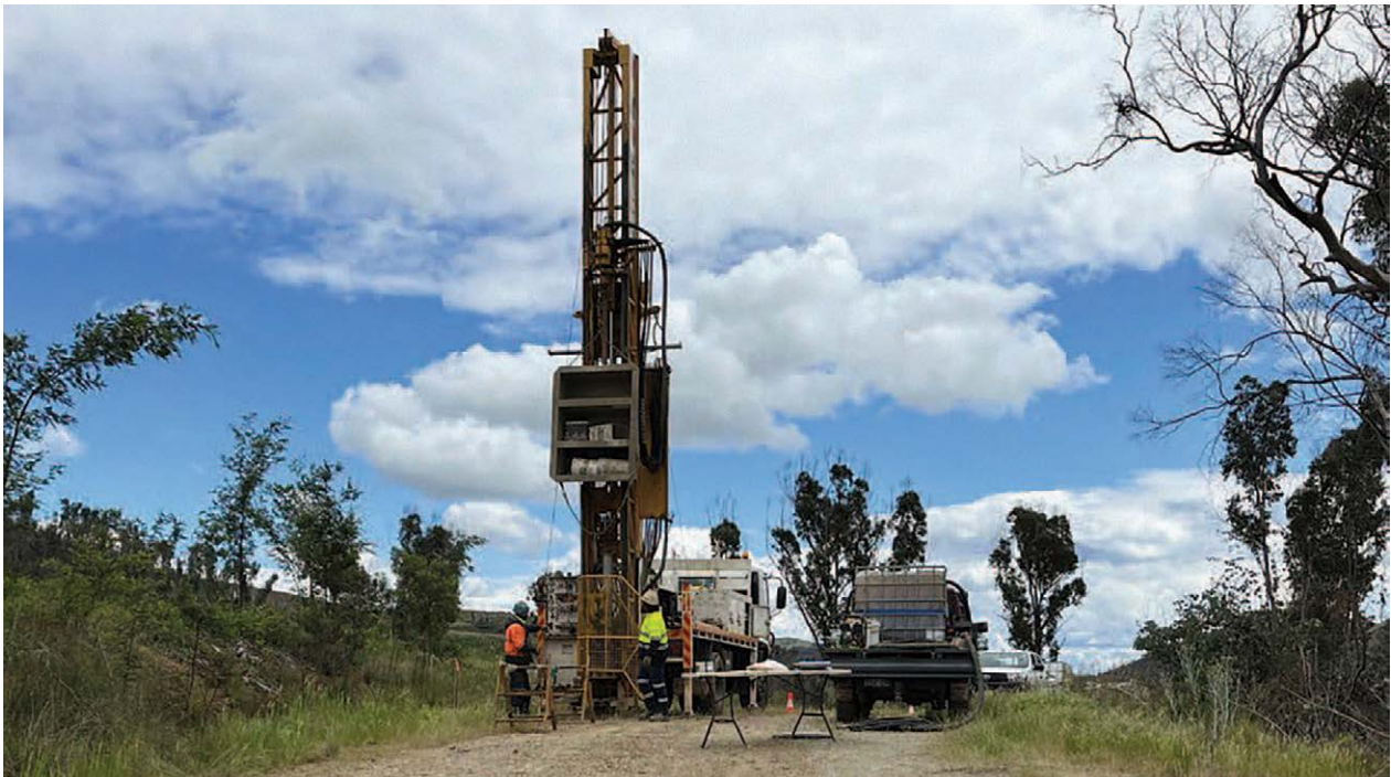
Pictured: Truck mounted drill rig collecting soil and rock samples on site.
