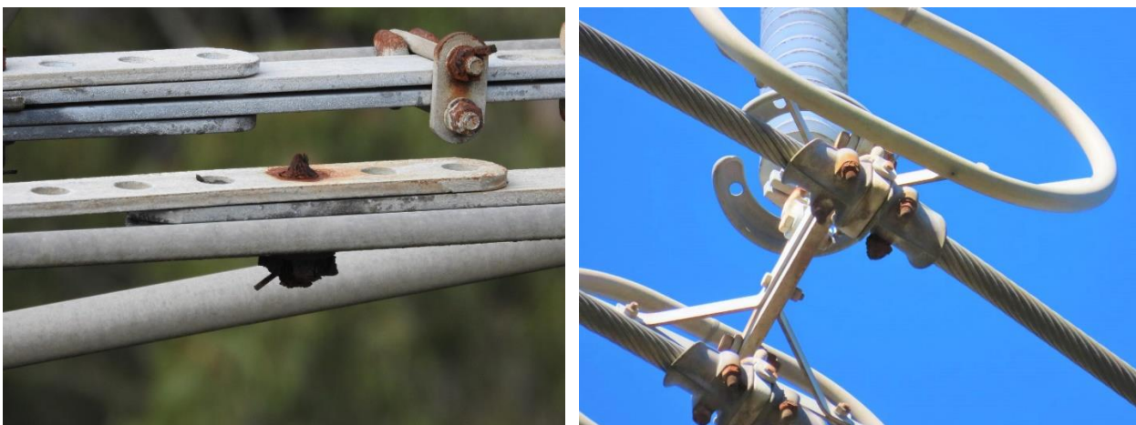
Figure 2-2 Corroded conductor fittings
