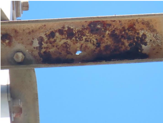
Figure 2-3 Corroded tower members
