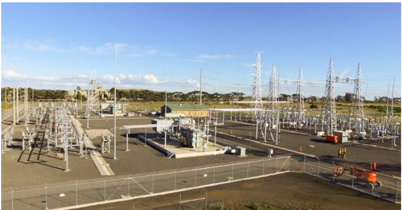
Figure 5 Deer Park 220kV and 66kV switchyard
