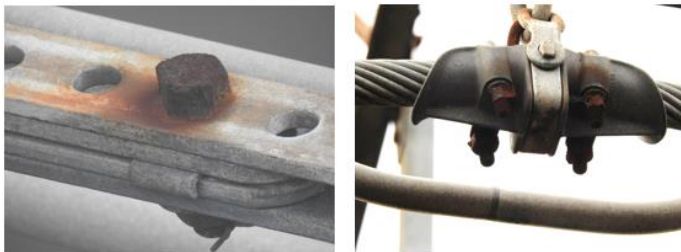
Figure 2-3 Corroded conductor and earthwire fittings
