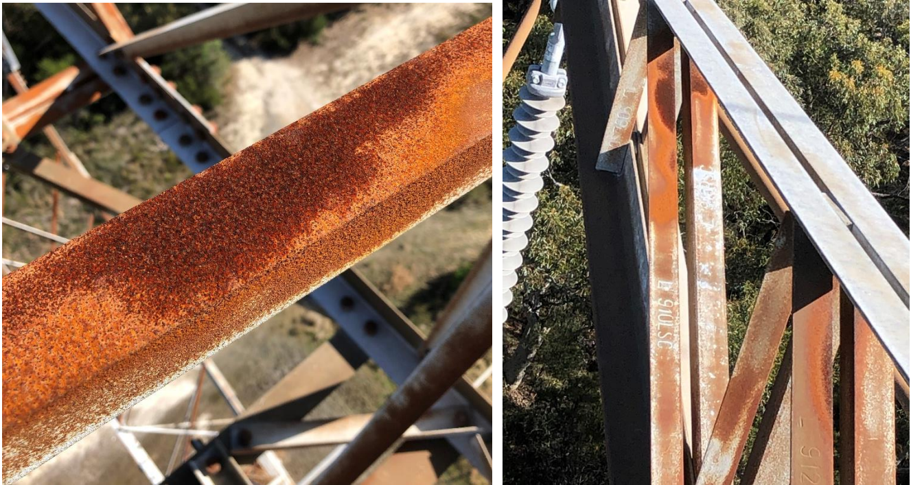
Figure 2-6 Corroded tower members
