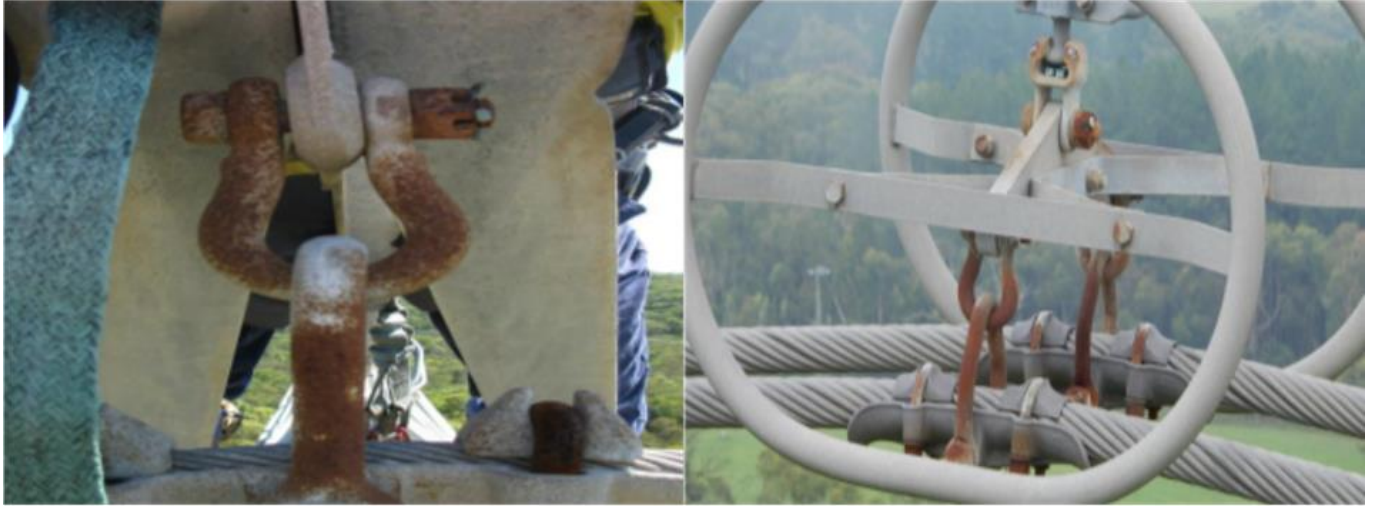
Figure 2-3 Examples of corroded components of Line 25 and Line 26: earthwire and conductor fittings
