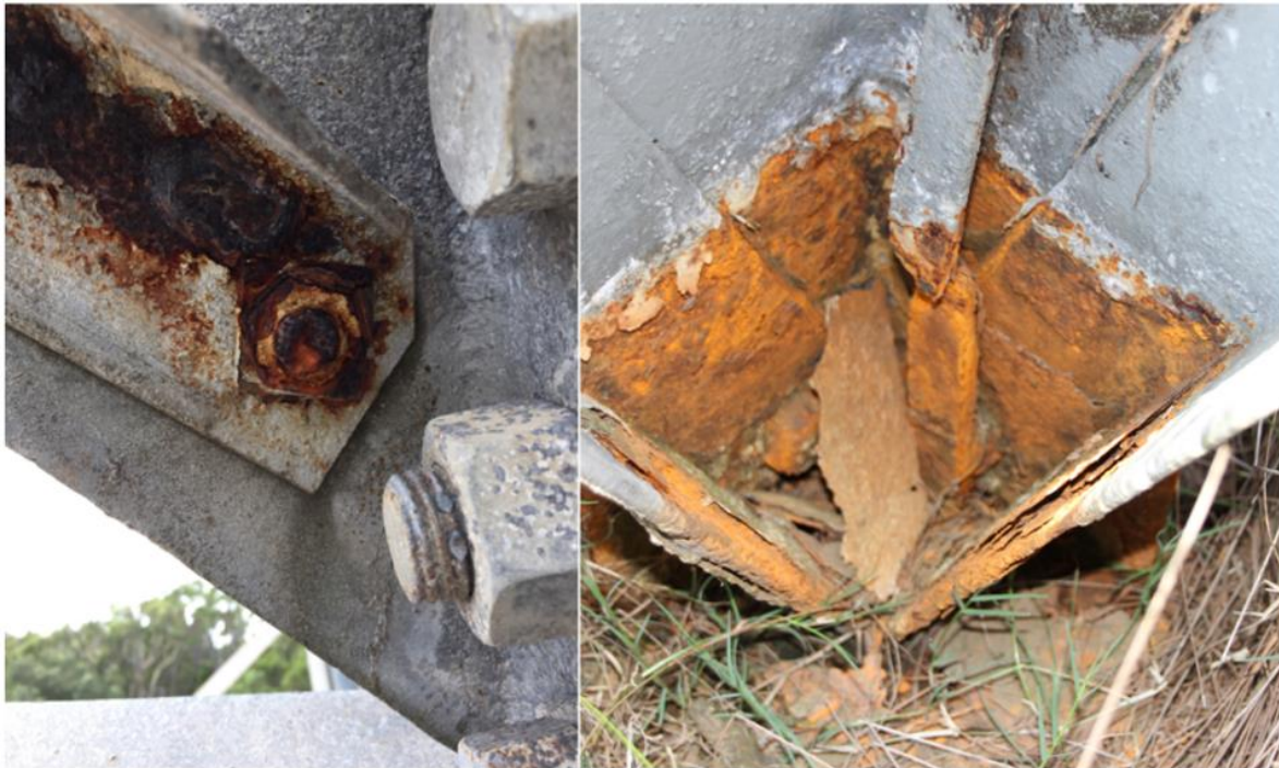
Figure 2-4 Examples of corroded components of Line 25 and Line 26: transmission tower steelwork and legs
