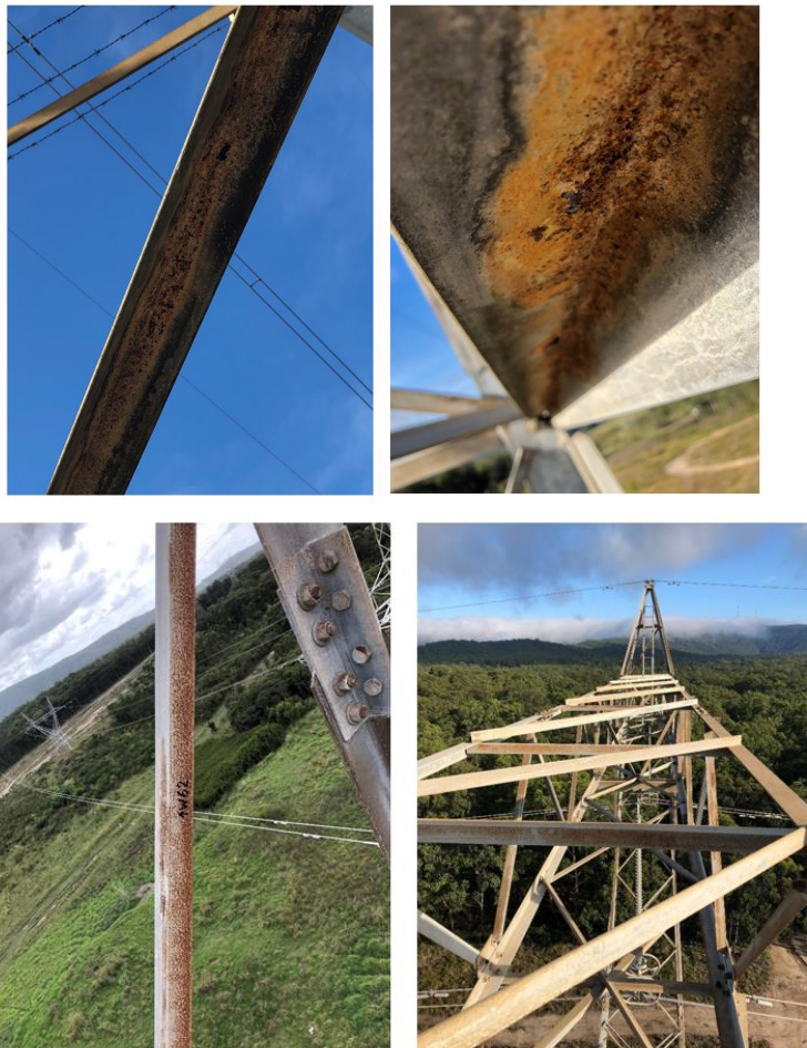
Figure 2-7 Corrosion affecting tower members
