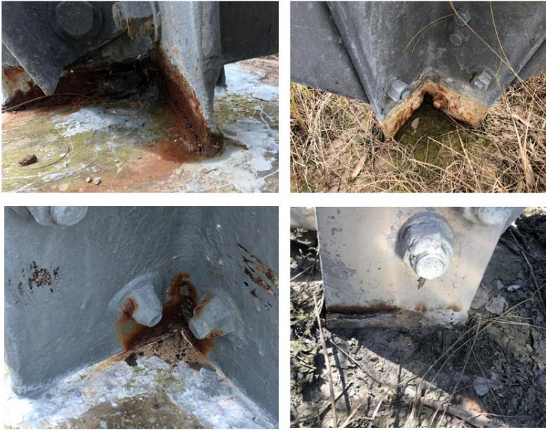
Figure 2-3 Corrosion affecting tower foundation at ground level
