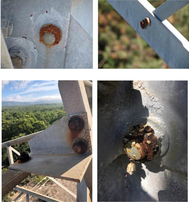
Figure 2-6 Corrosion affecting tower fasteners
