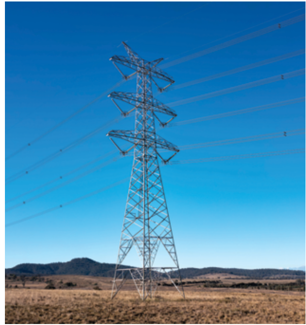
Pictured: Example of a 500 kV transmission tower.
