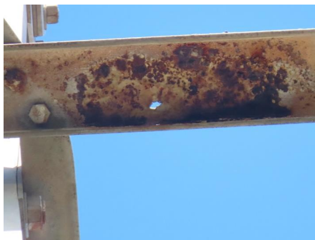
Figure 2.2 Corroded tower members
