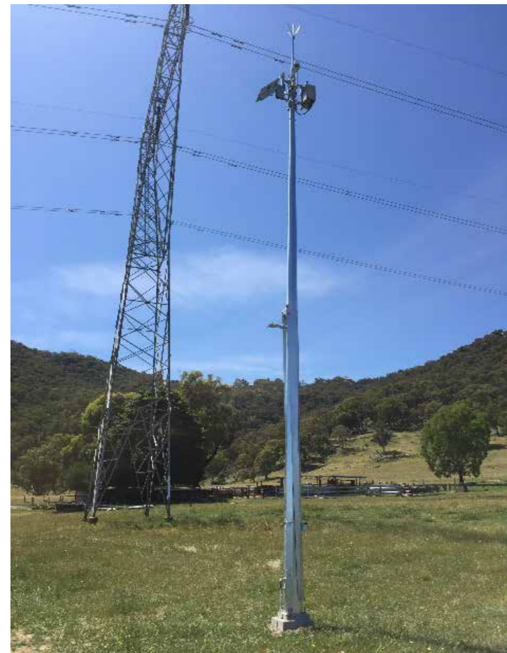
Figure 14-7: Dynamic line rating weather station
