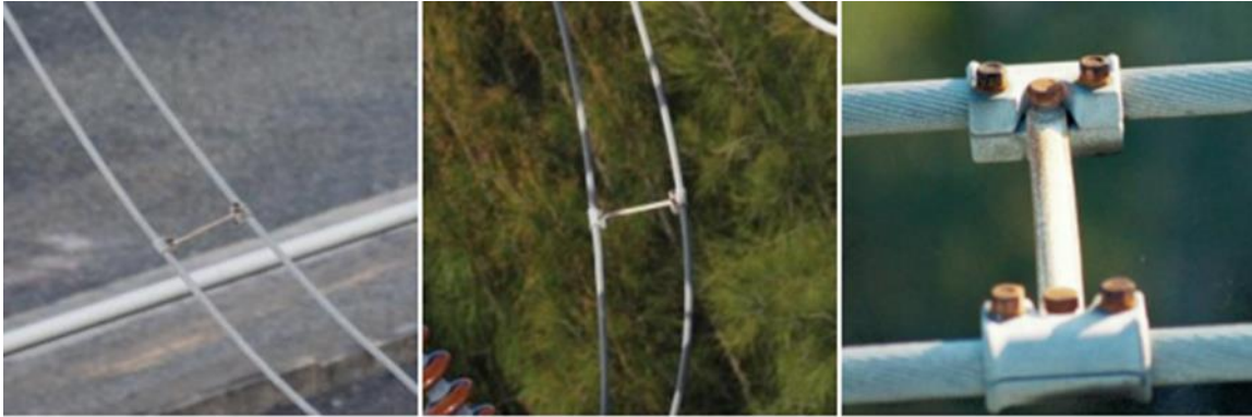
Figure 2-4 Corroded bolt and nuts of spacers
