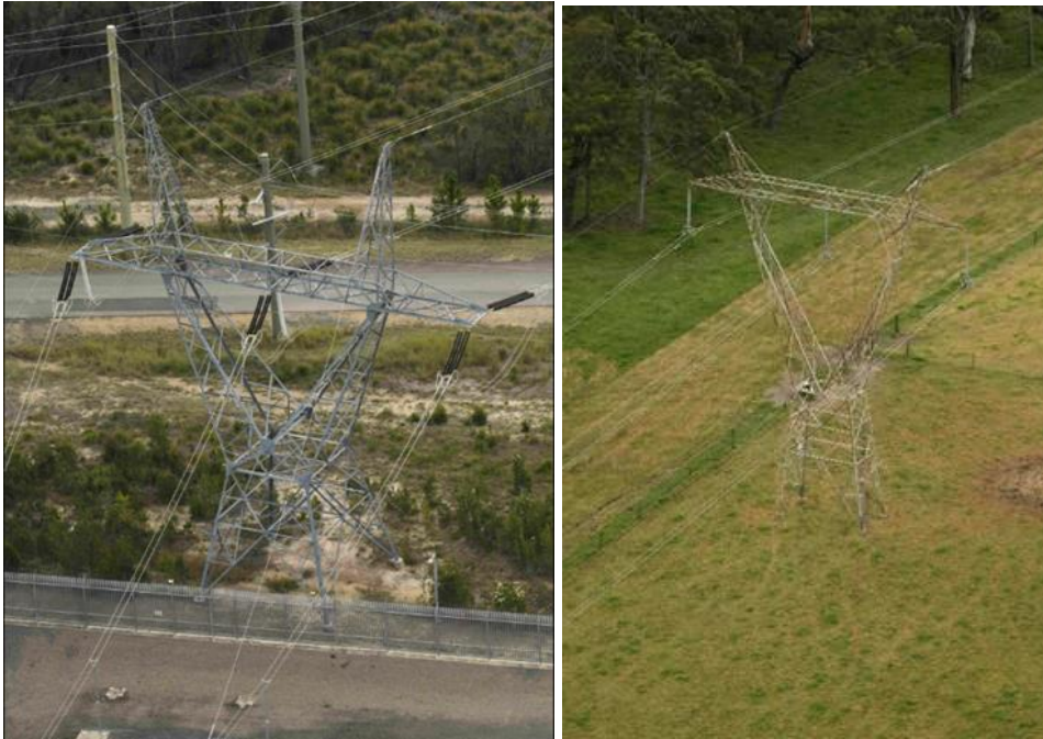
Figure 2-2 Line 23 tension tower (lefthand side) and suspension tower (righthand side)
