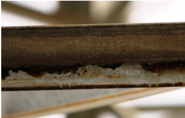
Figure 2-3 Corroded tower members
