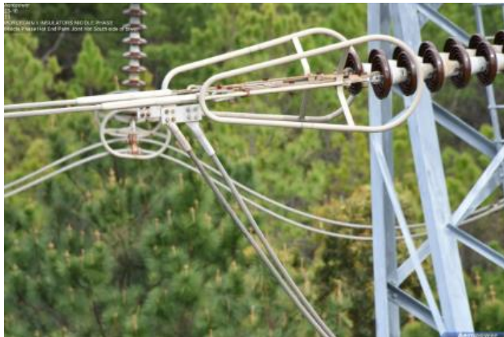
Figure 2-5 'Hotspots' 5 in the palm joint of conductors
