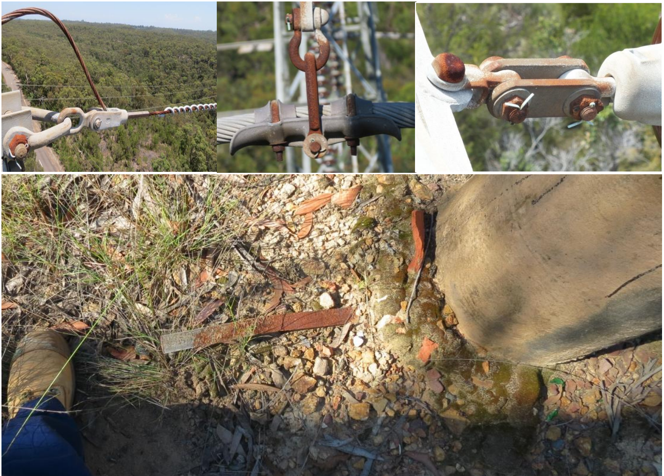
Figure 2-2 Corroded components of Line 959/92Z
