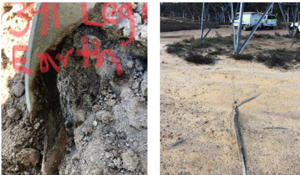
Figure 2-5 Tower earthing issues
