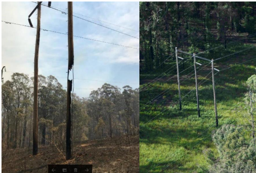
Figure 2-1: Damage caused to Line 963 in the November 2019 bushfires
