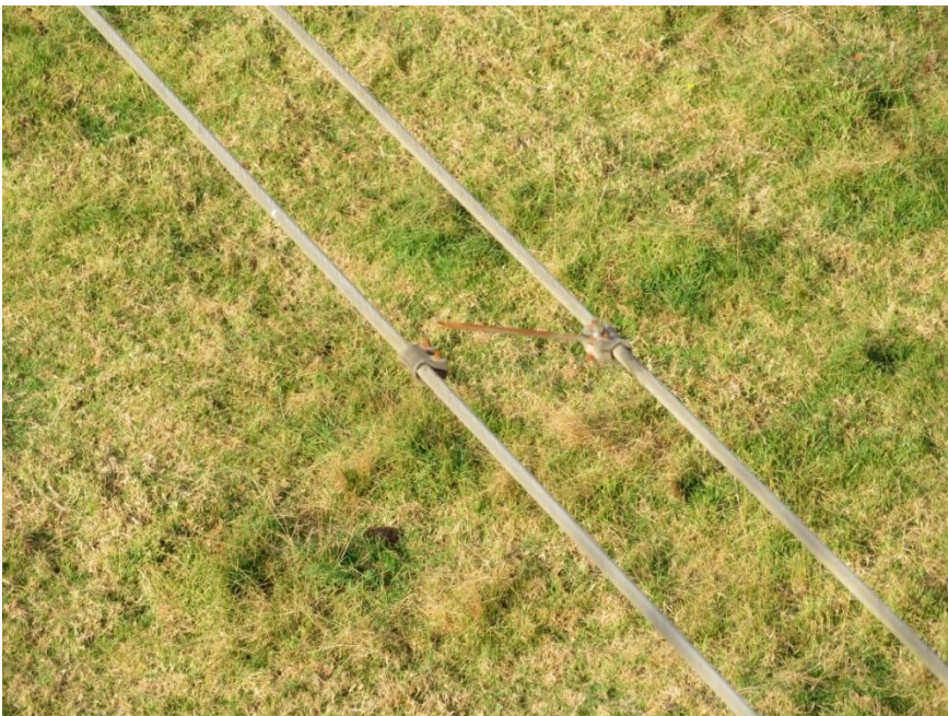
Figure 2-4 Damaged conductor spacers
