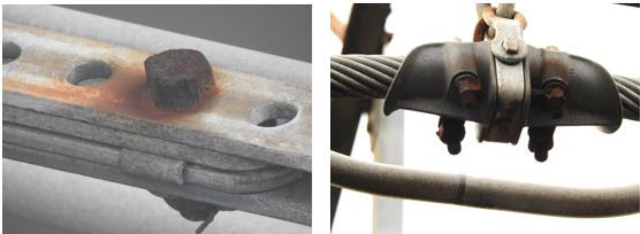
Figure 2-3 Corroded conductor and earthwire fittings
