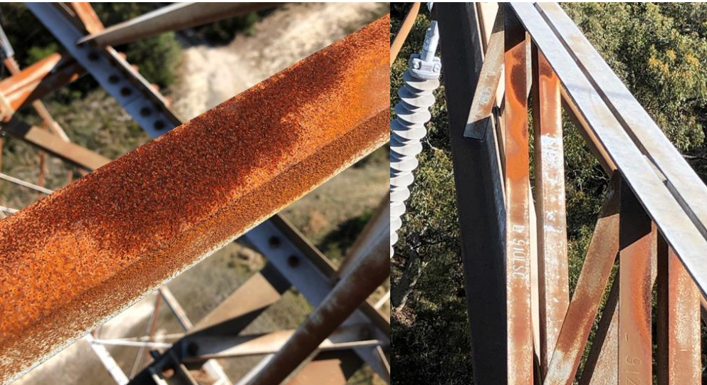
Figure 2-6 Corroded tower members
