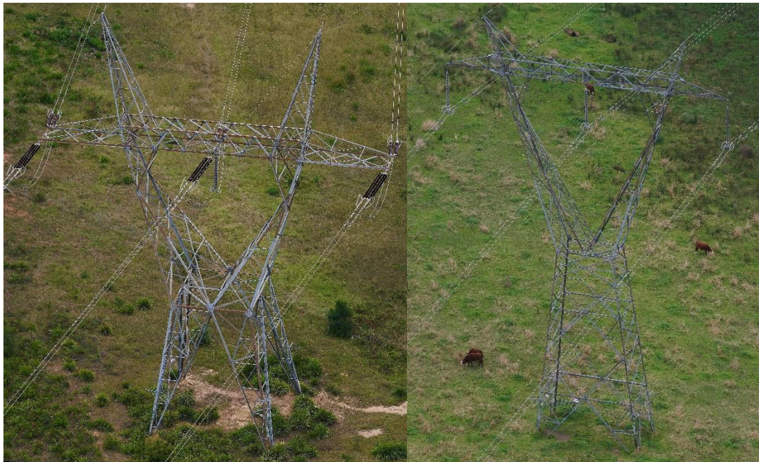
Figure 2-2 Line 16 tension tower (lefthand side) and suspension tower (righthand side)
