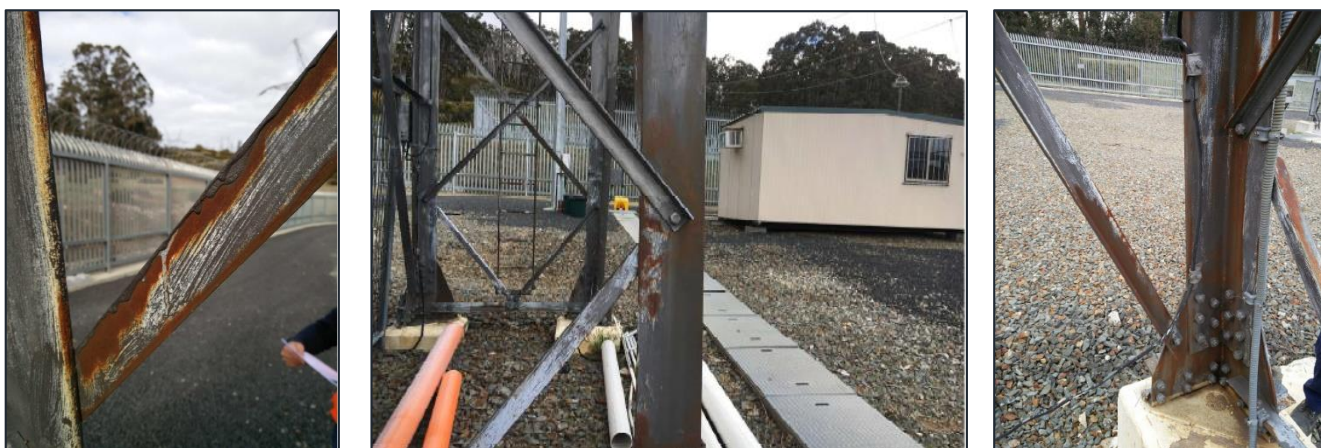
Figure 2-2 – View of gantry steel members showing corrosion
