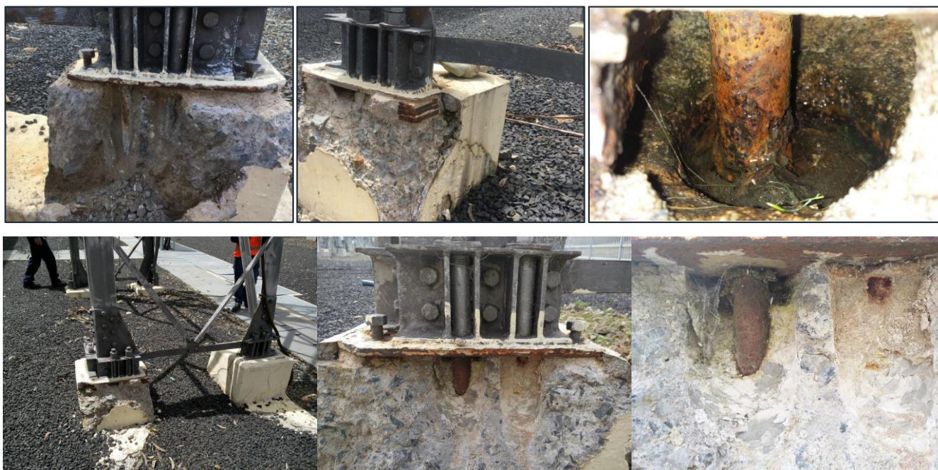
Figure 2-3 – View of corrosion to holding down bolts and baseplates
