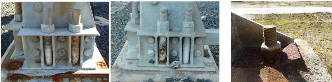
Figure 2-4 View of corrosion to holding down bolts and baseplates
