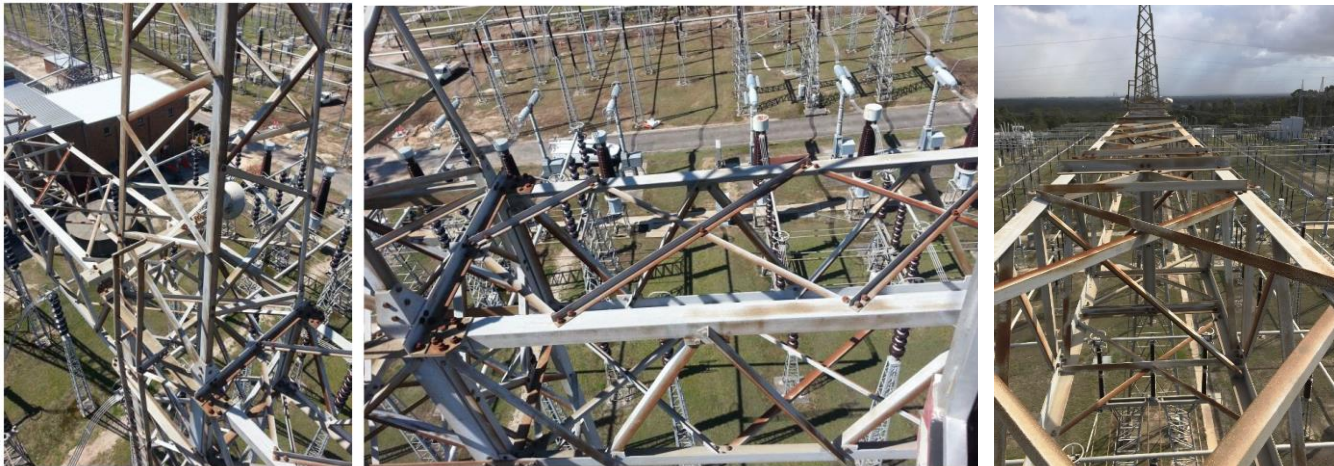
Figure 2-3 View of gantry steel members showing corrosion
