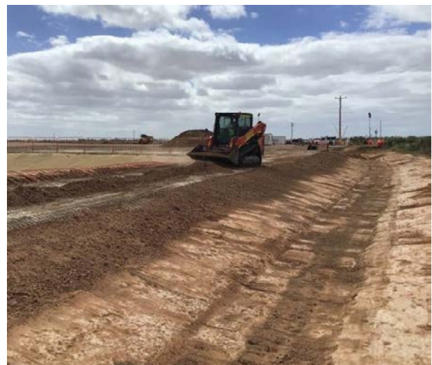
Pictured: Swale drain, similar to what may be built to manage water flow on HumeLink, being constructed on Project Energy Connect.
