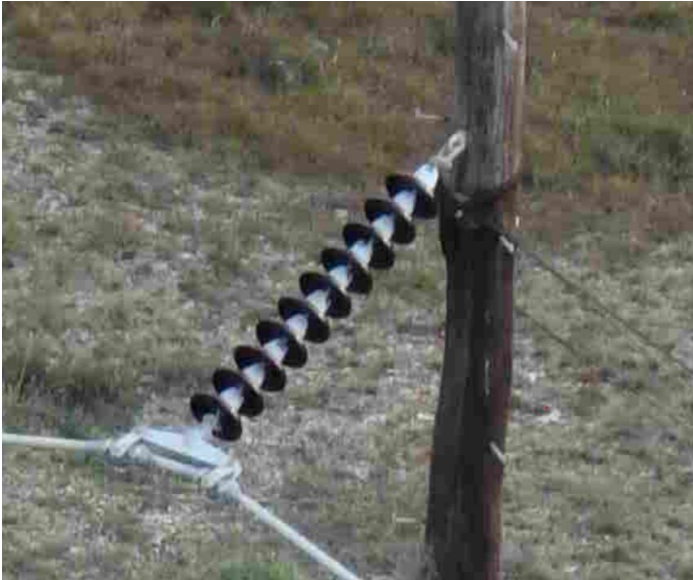
Figure 2-6 Insulator angle structure attachment eye-bolt pull through risk
