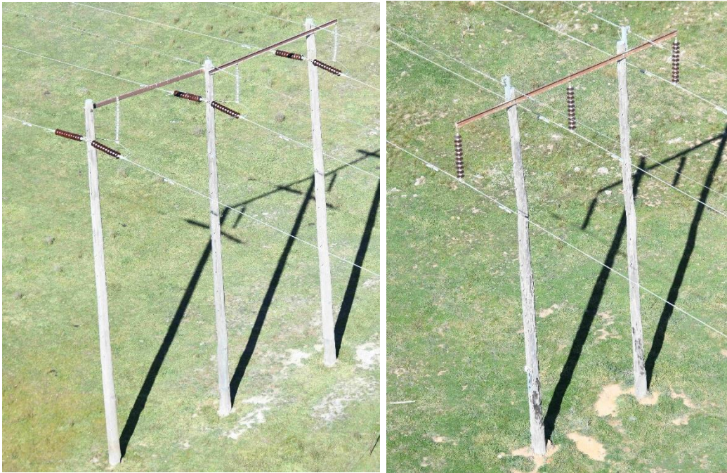
Figure 2-2 Line 977/1 tension wood pole structure (lefthand side) and suspension wood pole structure (righthand side)
