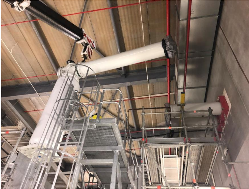
Rookwood Road Substation – installation of switching equipment
