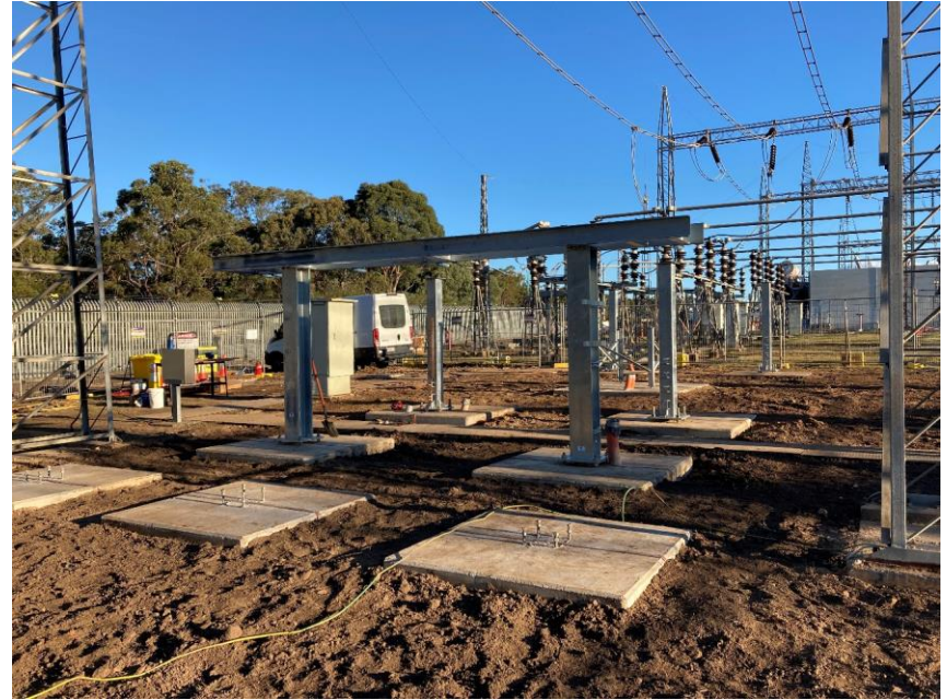
Sydney South Substation – HV equipment steel support structures
