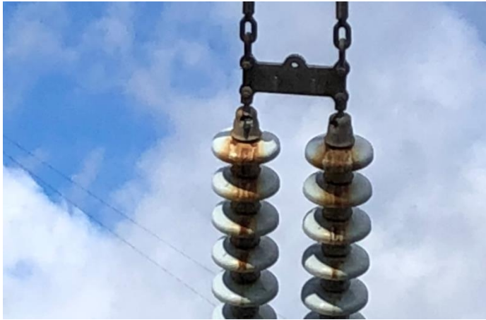
Figure 2-3 Corroded insulators and fittings
