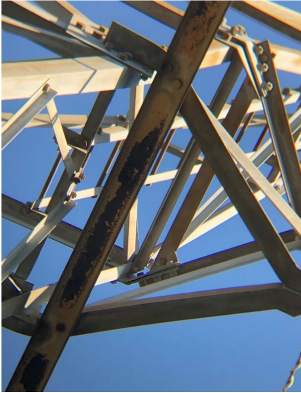
Figure 2-2 Corroded or bent tower members
