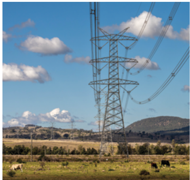
Pictured: Example of a 500 kV transmission tower.
