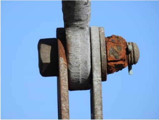
Figure 2-3 Corroded conductor and earthwire fittings
