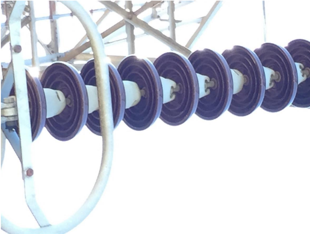
Figure 2-5 Rust on Insulator Pins
