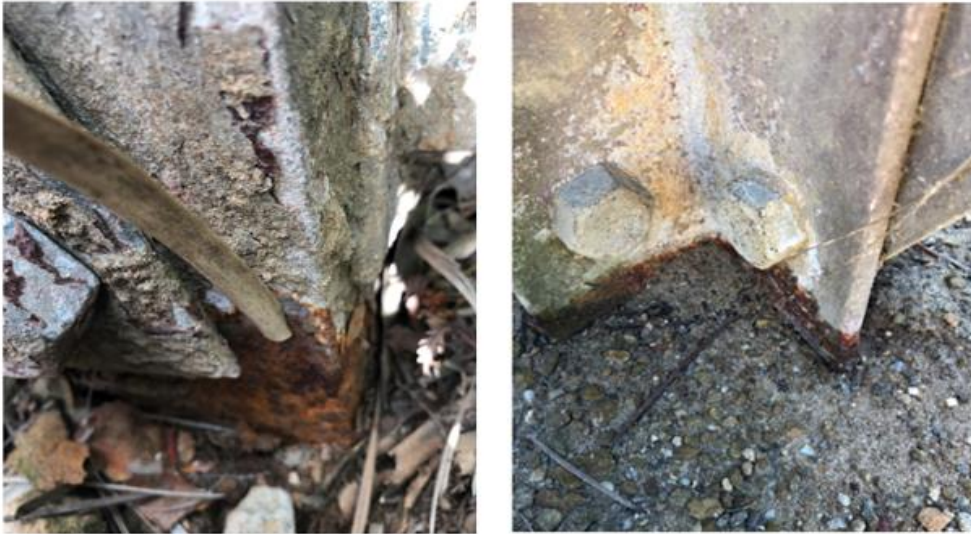
Figure 2-3 Corroded tower members
