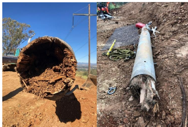
Figure 2-1: Example of wood rot on Line 86
