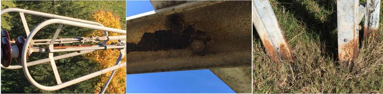
Figure 2-2 Examples of corroded elements of Line 8
