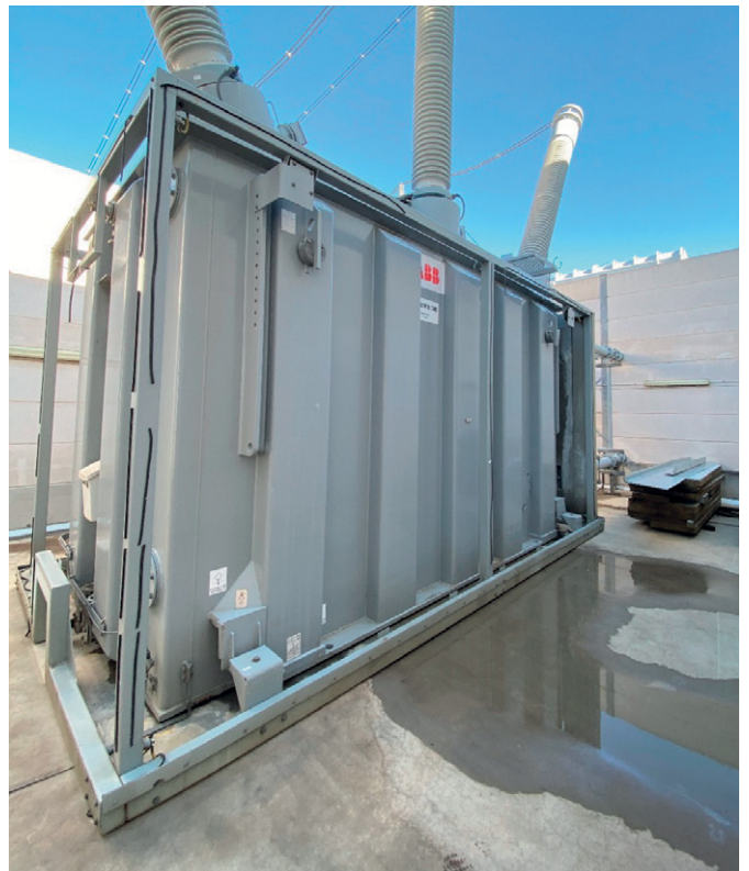
Image: A three phase 500kV shunt reactor.
