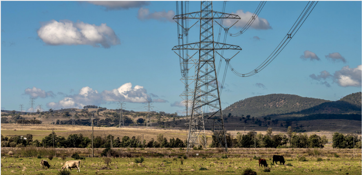
Pictured: 500 kV transmission towers in Muswellbrook, similar to those that will be built on HumeLink.
