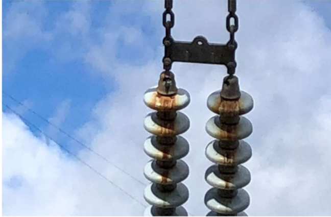
Figure 2-3 Corroded insulators and fittings
