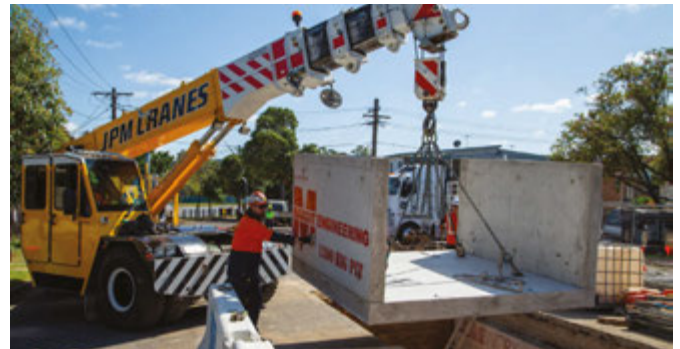
电缆接驳井建筑 (Hillcrest Avenue, Greenacre)
