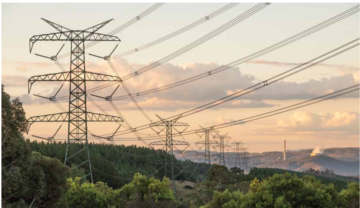
500 kV double circuit transmission lines
