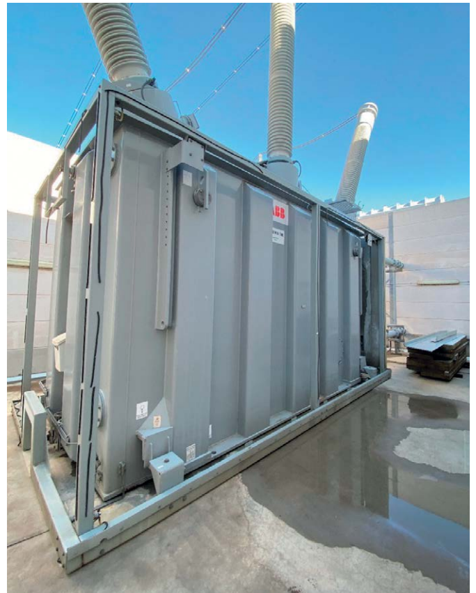
Image: A three phase 500kV shunt reactor.
