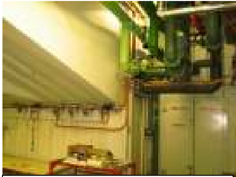
Rm 7.01 – Existing Air Handling Unit
