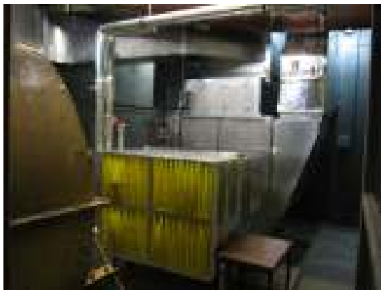
Rm 7.06 – DICER 2 – Main Installation
