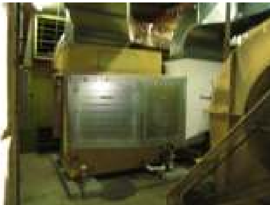
Rm 7.01 – DICER 1– Main Installation
