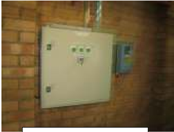
Rm 7.01 – DICER 1 Control Panel
