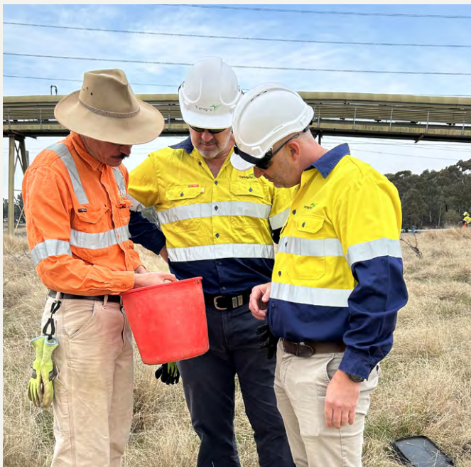
Images: Ozark and members of the Transgrid project team on site for test excavations.
