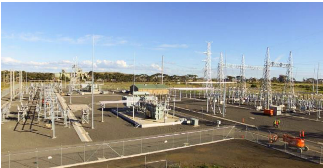
Figure 6 Deer Park 220kV and 66kV switchyard
