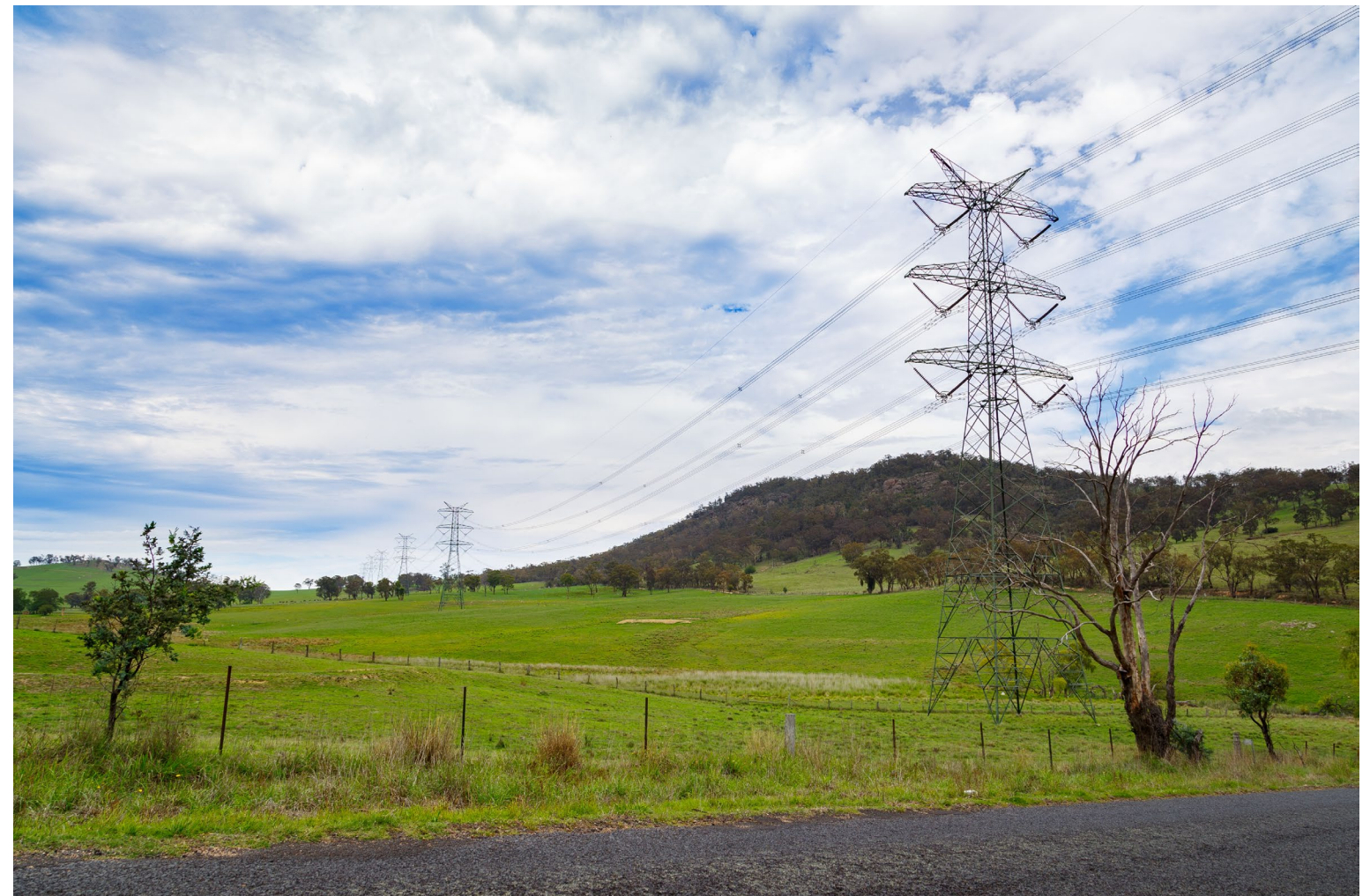
500kV transmission line near Tarana
