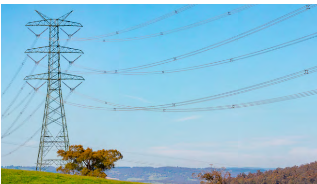
Image 1: Example of a 500 kV transmission line structure.
