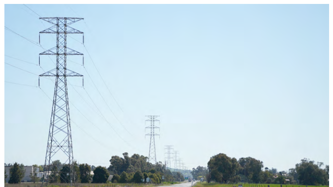
Image 2: Example of a 330 kV transmission line structure.
