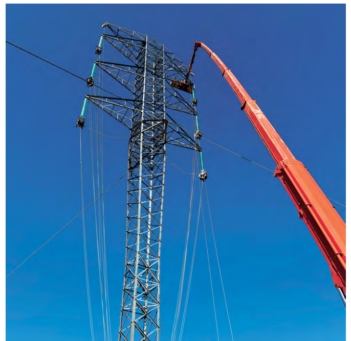
Image 5: Example of a stringing of a 500kV transmission tower from the EnergyConnect (NSW) project.
