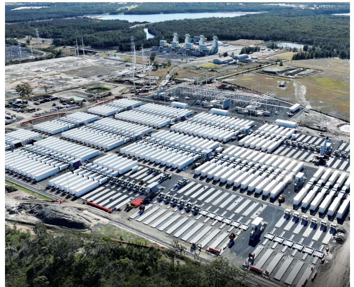
Waratah Super Battery (courtesy of Akaysha Energy)
