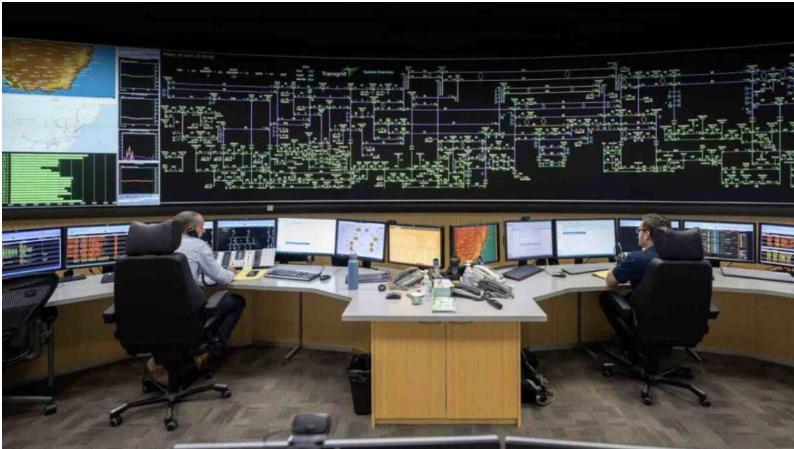
Figure 2-3: Transgrid's system control room and current information and monitoring capabilities
