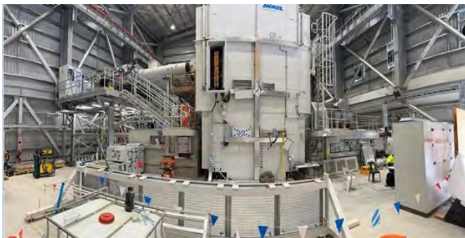
Image: Buronga substation testing
