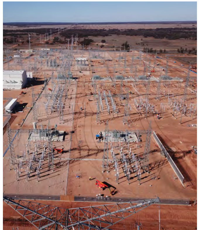
Image: Buronga Substation in May 2024.
