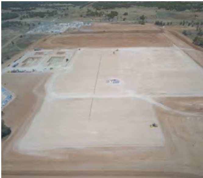
Image: Buronga Substation in February 2023.
