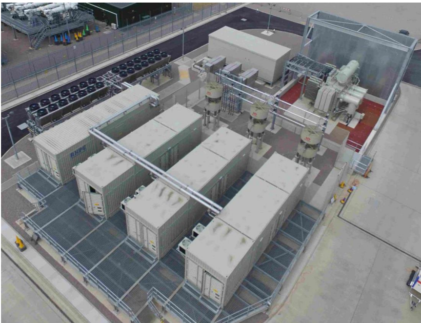
Photograph 1 Indicative STATCOM equipment
