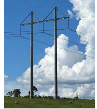
Pictured: An example of a two pole configuration.
