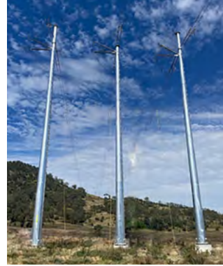
Pictured: An example of a three pole configuration.
