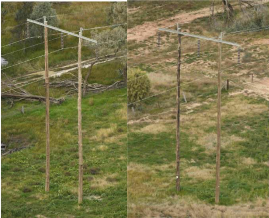
Figure 2-2 shows wood pole structures on Line 94U.
