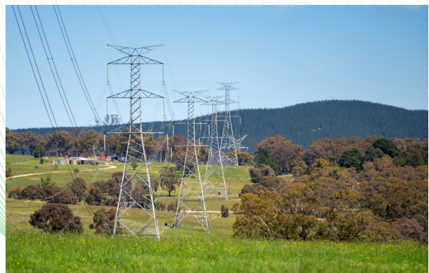
Transgrid's existing 330kV line near Wallerawang
